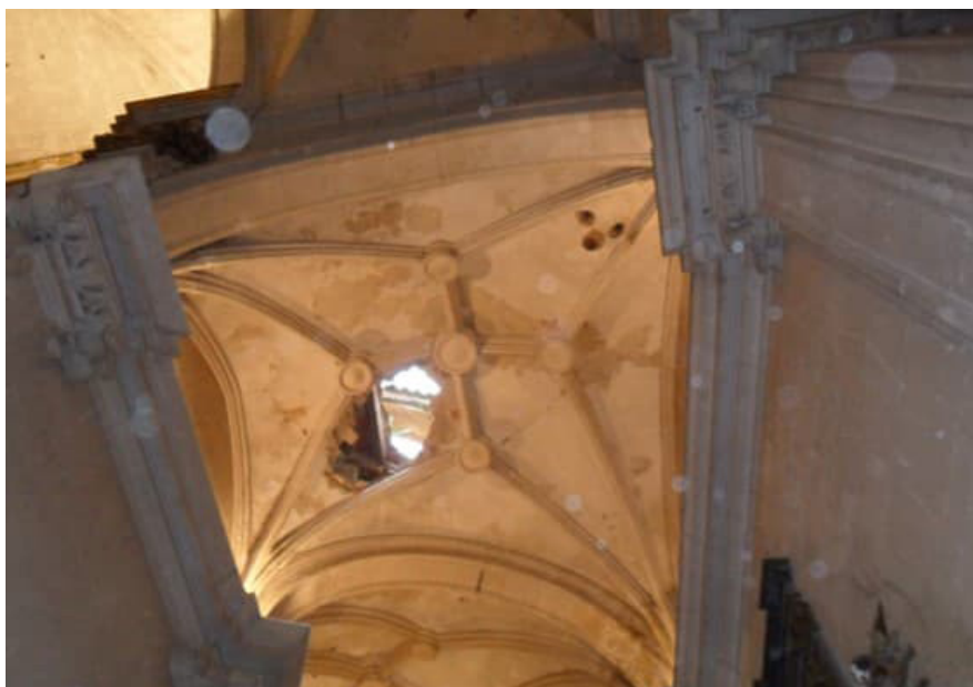
Figure 6. Former St. Patrick's Collegiate Church. Plainly visible damage in the interior. Hole in the double curvature vault.
