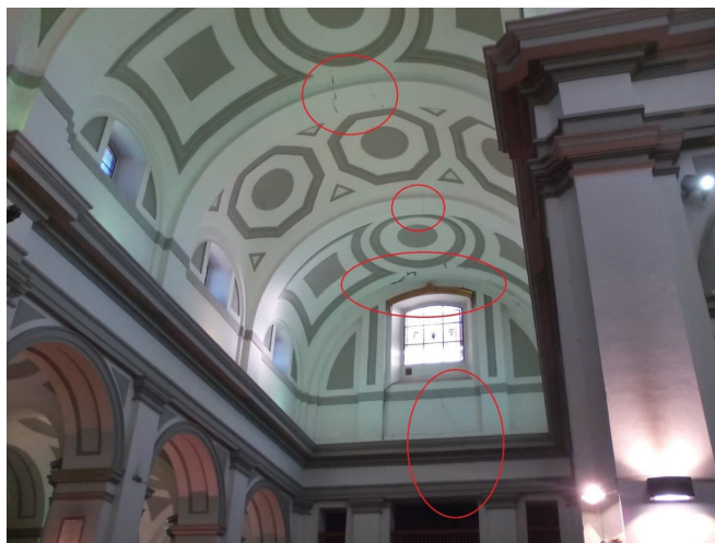
Figure 7. Parish Church of the Incarnation in Santa Fe. Longitudinal cracks in the claddings of domes, vaults, arches, and vertical walls.
