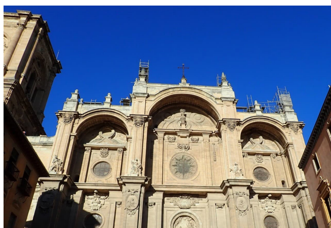
Figure 8. Granada Cathedral. Auxiliary emergency measures, removal of ornamental elements from the façade.
