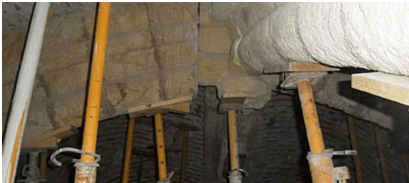
Figure 1 1 . Photograph of the interior of the Espolón Tower [Tower on the Spur] of the Castle in Lorca after the 2011 earthquake.
