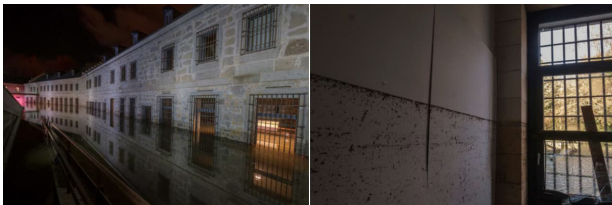
Figure 12. Flooding of the lower patio and the water level mark after the 2020 event.
