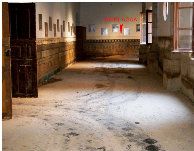
Figure 5. St. Francis' Convent. Accumulation of mud on stone walls and floors and damage to wall cladding, paintings, and woodwork.
