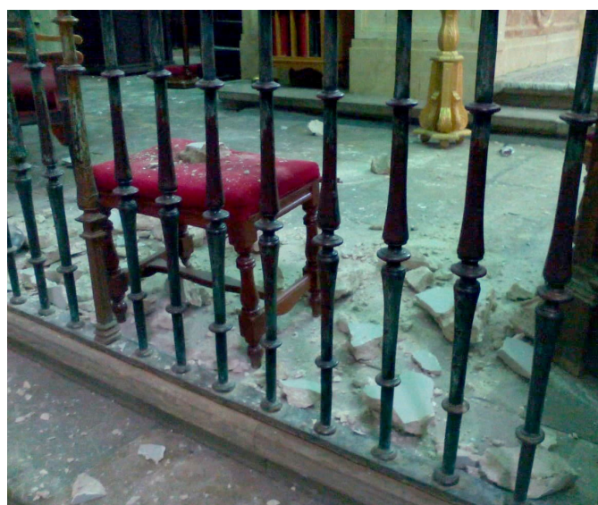
Figure 4. Fallen masonry cladding in the Santa Fe Parish Church of the Incarnation. These can be seen to be quite thick, typical for buildings of this kind.
