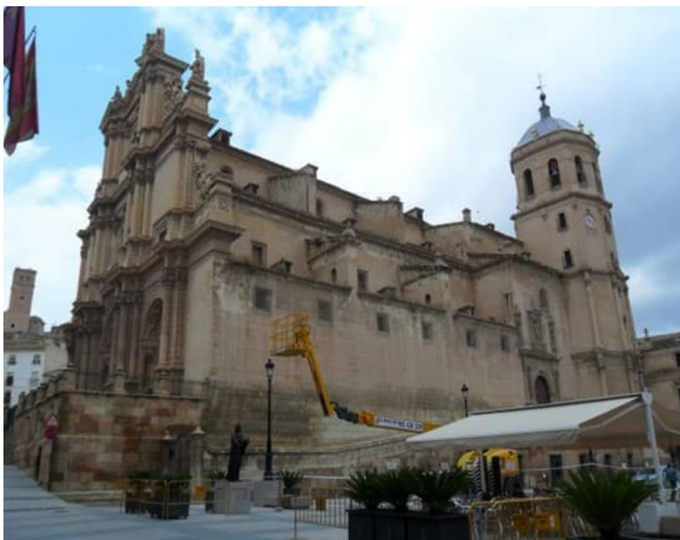
Figure 2. Photograph of the former Saint Patrick's Collegiate Church showing one of the cranes used to remove elements from the upper portions on the building that were at risk of falling.
