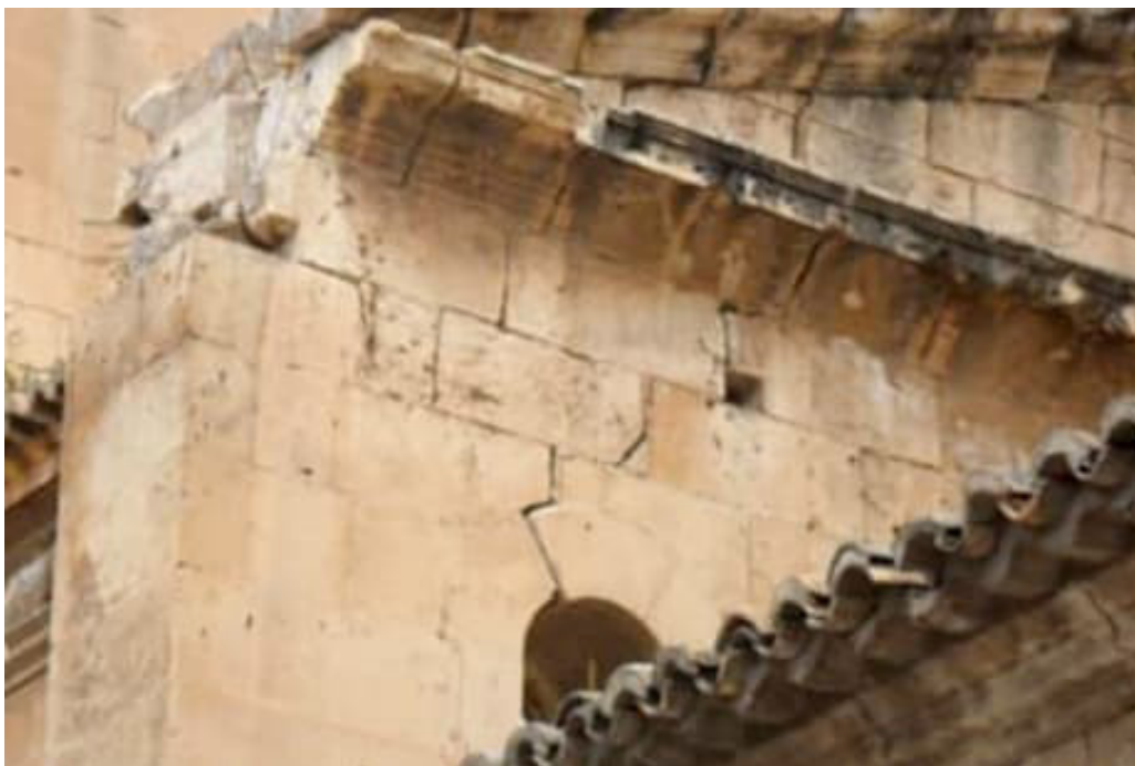
Figure 3. Photograph showing damage plainly visible from the exterior. The pinnacle on the end of the buttress and part of the cornice have collapsed. There is a crack over the arch located in the wall section of the buttress itself, and the keystone has dropped down. Plants can also be seen to be growing on the roof, an indicator of inadequate maintenance.
