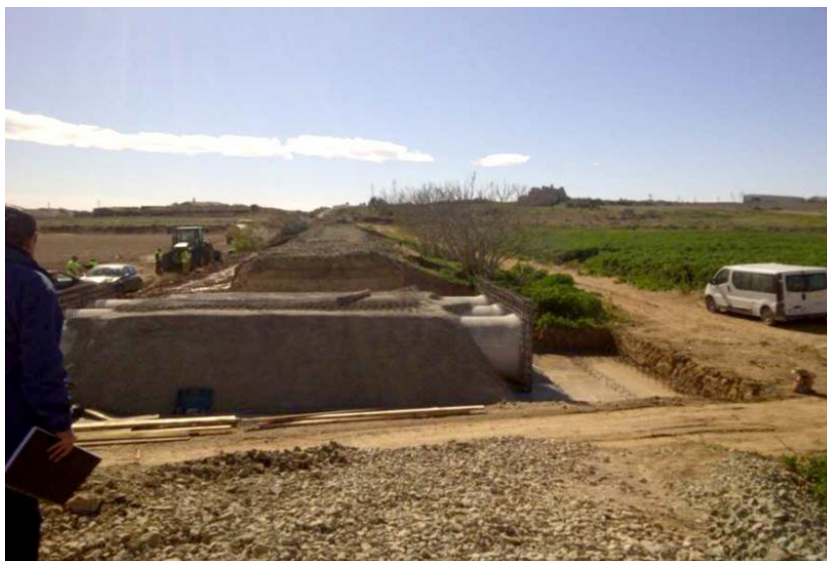
Figure 7. Execution of new drainage works on the Murcia-Águilas railway line due to shifting of drainage channels following the 2012 flooding.
