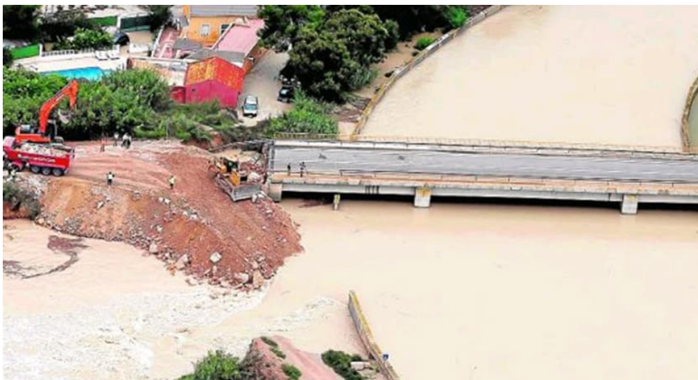
Figure 12. Breakage of the channelling of the river Segura at Almoradí. Source: Segura River Basin Authority.
