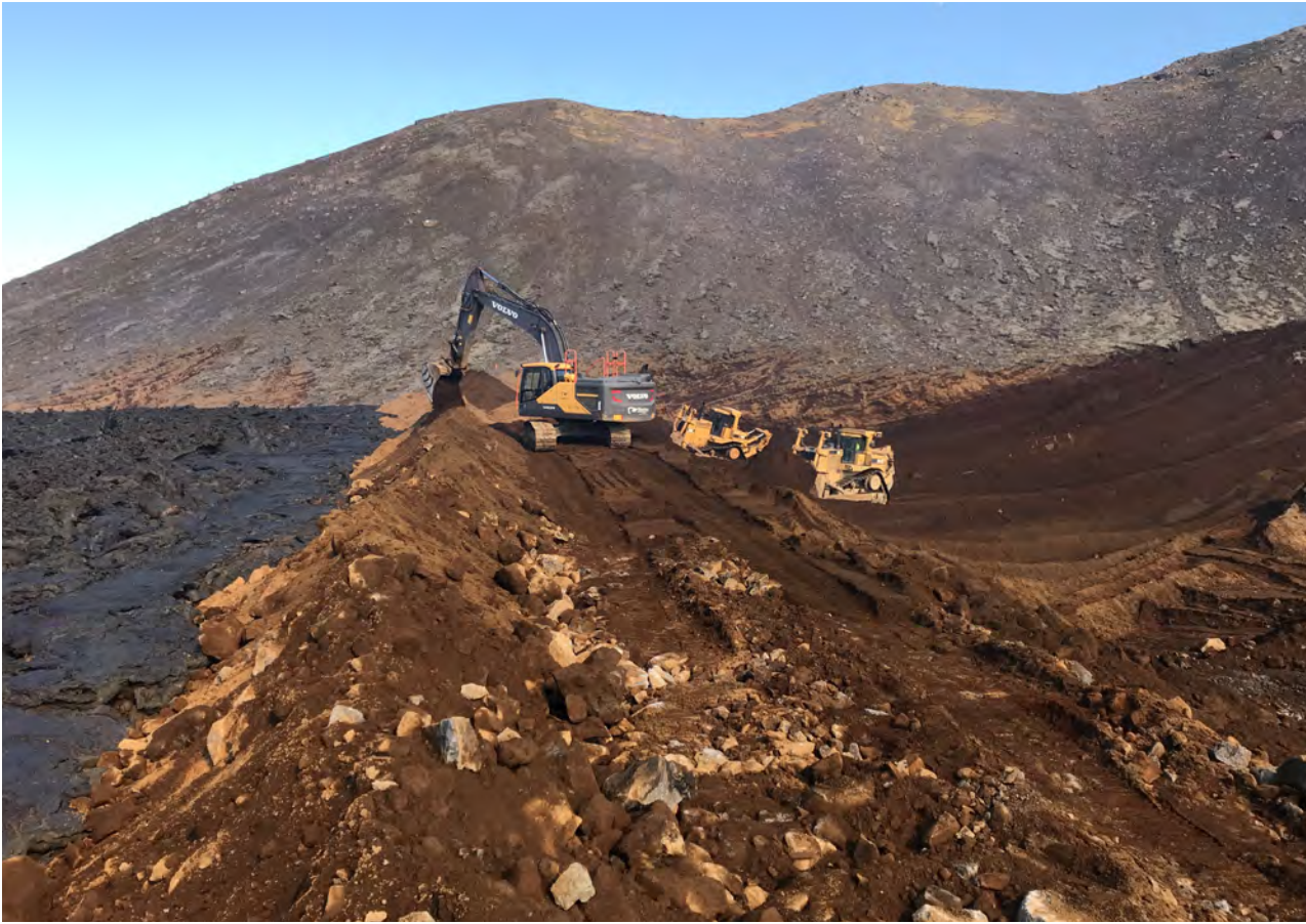
Figure 7. Emergency heightening of the eastern dam, one day before overtopping. Source: Photo by Ari Guðmundsson.
