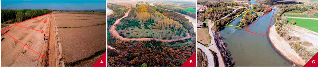
A. Setting back a dyke in Alfaro (LR) 710 m. River Ebro. B. Dyke removal at Cabañas de Ebro (Z). C. Novillas (Zaragoza). Work on vegetation and obstructive elements. River Ebro.
