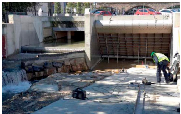
Setting up caissons at the confluence of the rivers Queiles and Ebro. Tudela (NA).
