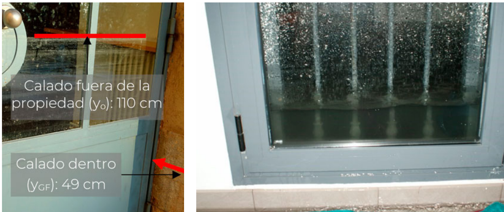
Figure 8. High-water marks following a flood event both inside (49 cm) and outside (110 cm) a property.
