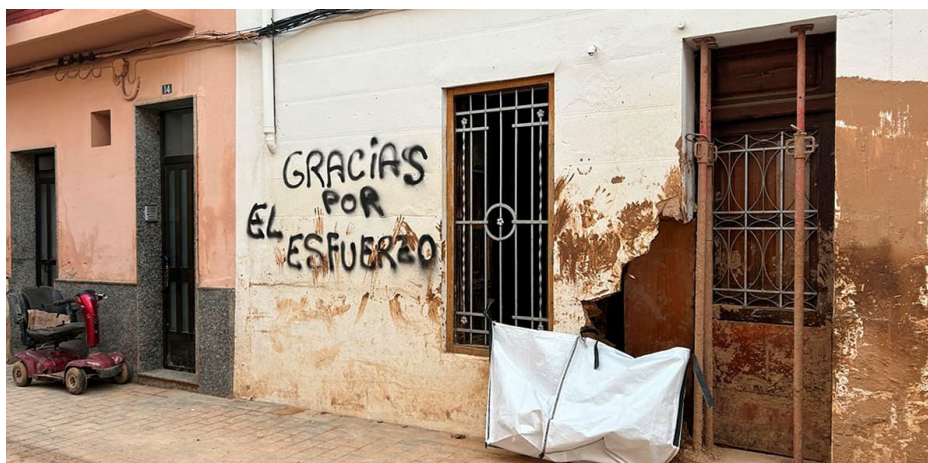
Image 5. Inundated home façade in Paiporta, with a graffiti reading “Thanks for your efforts”. Source: Consorcio de Compensación de Seguros.
