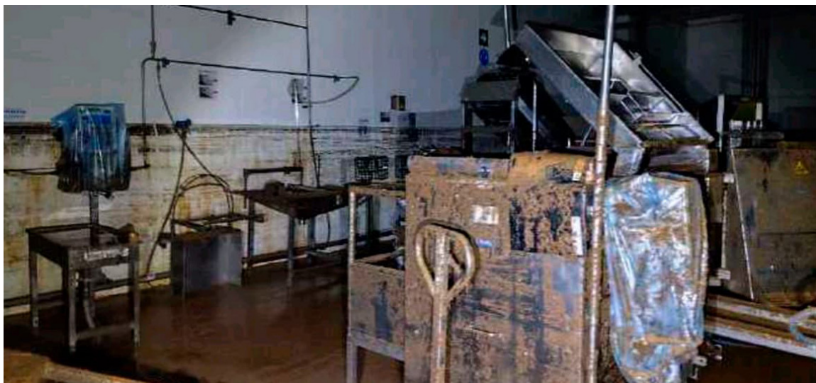
Image 10. Damaged food industry plant in Torrent. Source: Consorcio de Compensación de Seguros .
